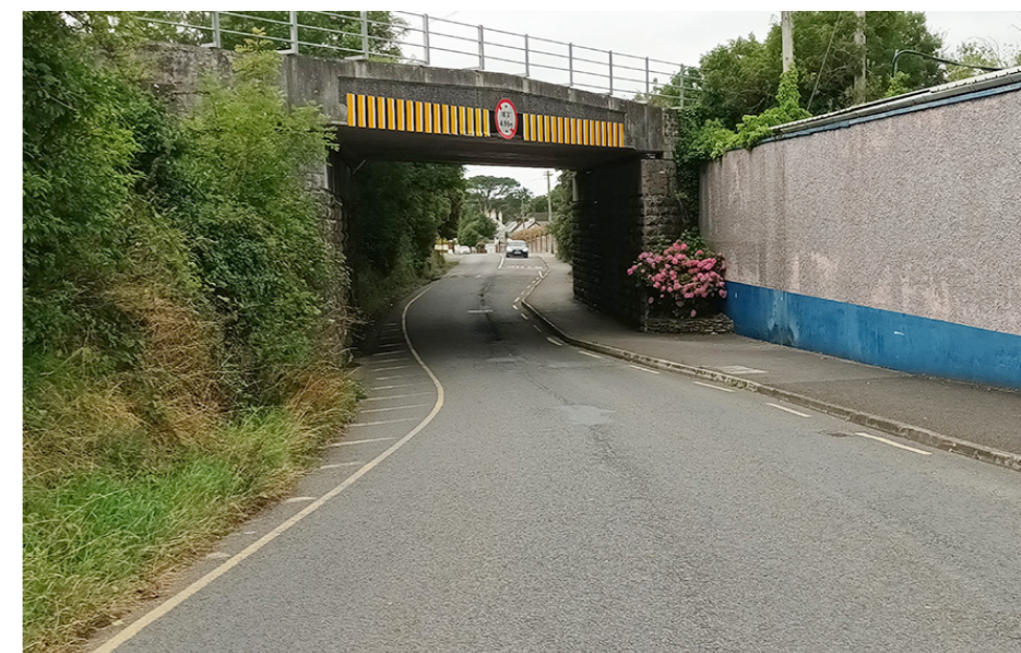
Fig.23 - Image of railway viaduct over Barn Road with narrow footway and one-way carriageway.
