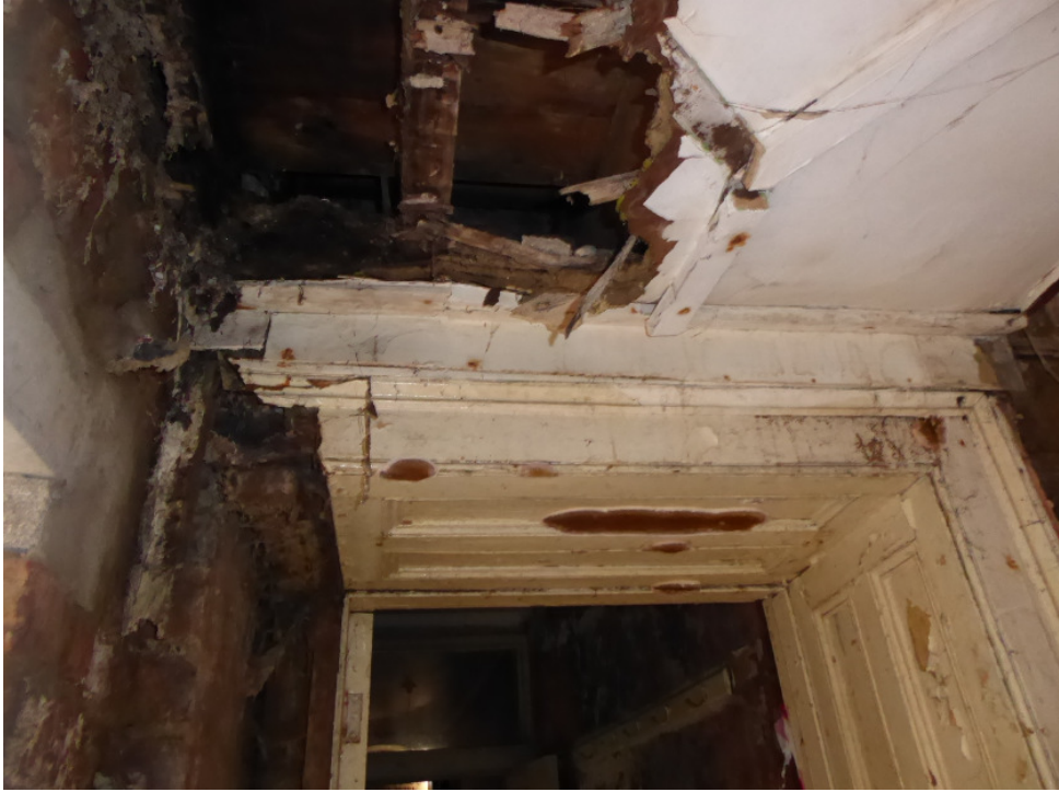
Fig 2.11 – Significant loss of internal joinery-work at the Judges' Chambers.
