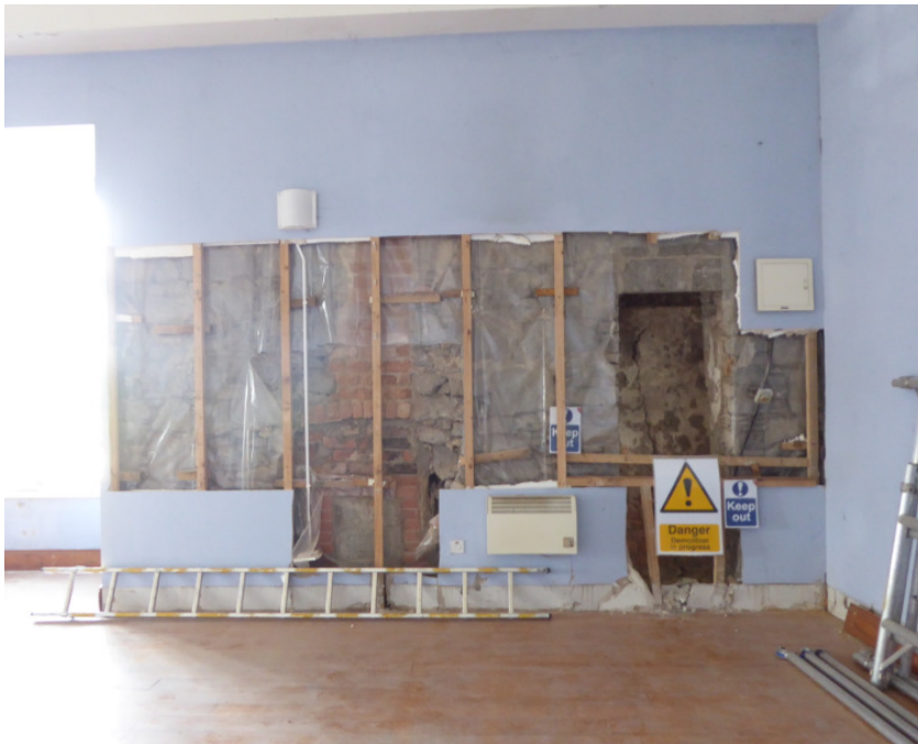
Fig 5.16 – Garderobe can be seen on the RHS where it was concealed behind plasterboard lining.
