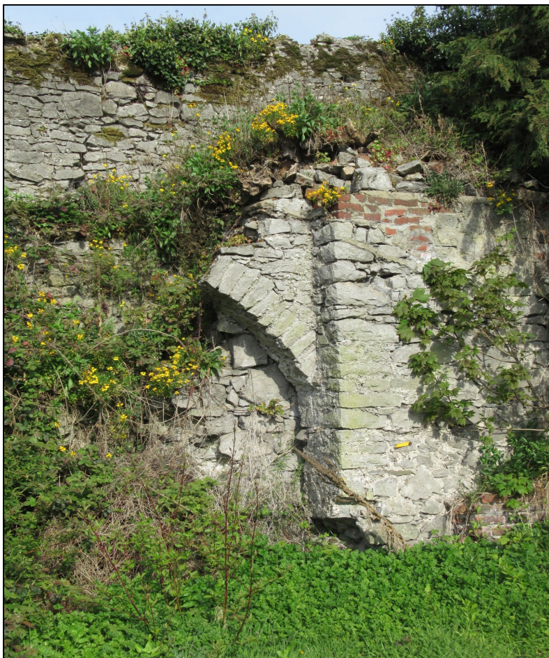
Photo 3: Detail view showing the current conditions on the east side of the town wall. Note the extent of invasive vegetation, missing mortar joints, structural cracks, and undermining of the wall's base.
