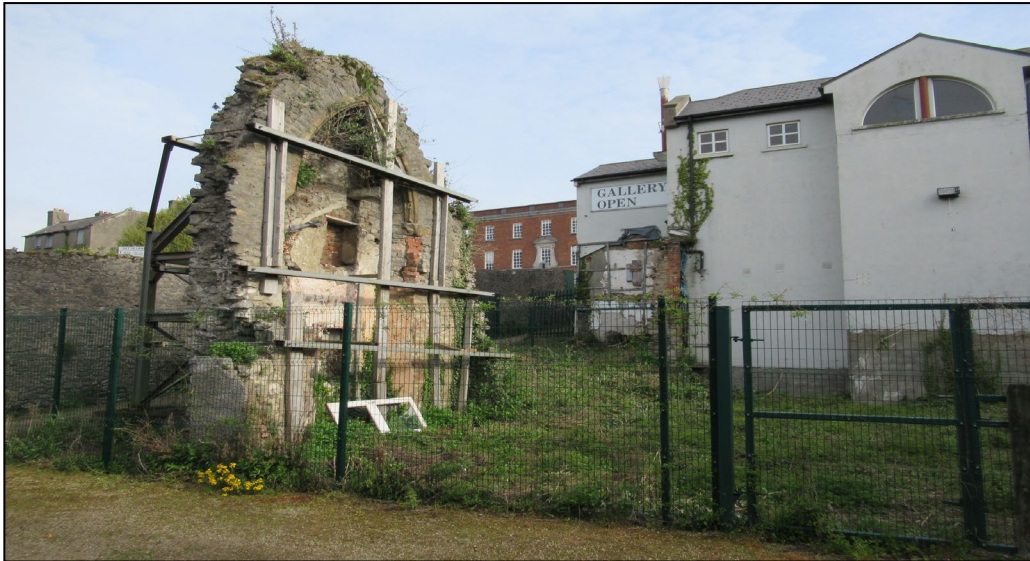
Photo 8: General view showing the west gable end that survives from a side chapel at The Old Abbey (St Mary d'Urso). This fragment of the chapel was uncovered during the late 20 th century when later structures were removed. It is currently in a precarious structural condition and depends on temporary props for its stability.
