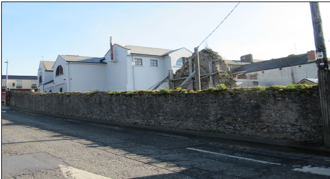
Photo 5: General view looking north-east, showing the free-standing west gable from the side aisle of the chapel at the Abbey of St. Mary d'Urso. The C19th rubble stone boundary wall running along the edge of Father Connolly Way is shown, forming a solid boundary between the road and the end of Old Abbey Lane.
