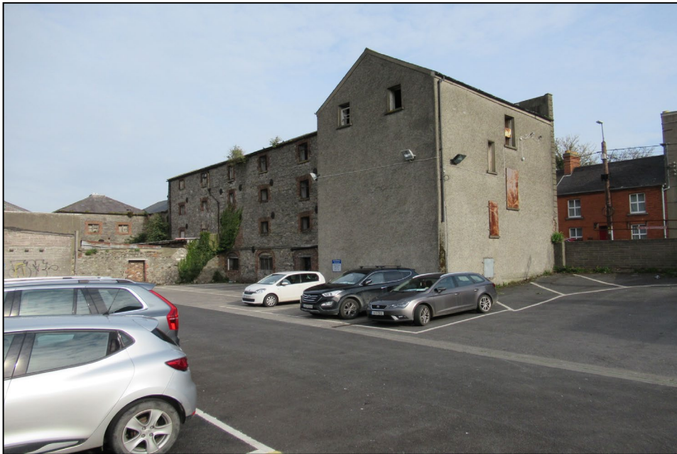
Photo 20: General view showing the south elevations to the unused structures in the previous photo, and the open space to their rear.
