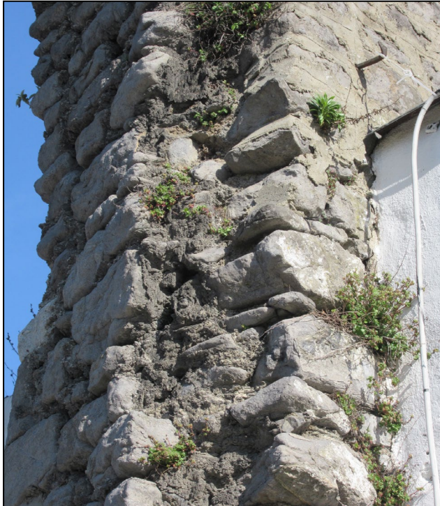
Photo 7: Detail view showing the fragile masonry on the underside of the arch at the base of the medieval tower at The Old Abbey (St Mary d’Urso). Careful conservation works are required to all of the upstanding masonry ruins from the abbey, to prevent further deterioration.
