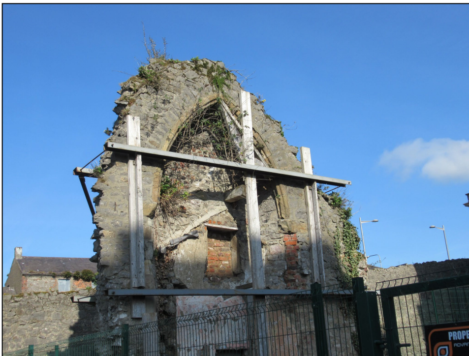
Photo 9: Detail view showing loose masonry on the west gable that survives from the Abbey of St. Mary d'Urso.
