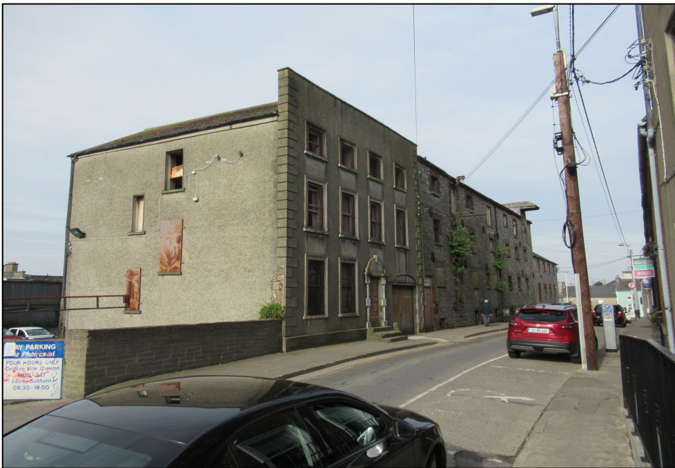
Photo 19: General view showing a derelict group of structures on the south side of the western end of Fair Street, immediately behind Barlow House. At left is a large house dating from the
