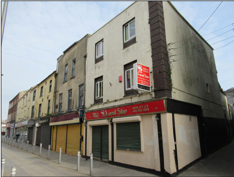
Photo 16: General view showing a row of former houses on the north side of West Street, in varying conditions and showing signs of dereliction and lack of maintenance. Barlow house is just beyond the left end of this group of 18 th century structures.
