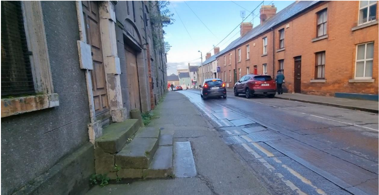
Figure 81: Steps presenting trip hazards in footway and obstructing footway width
