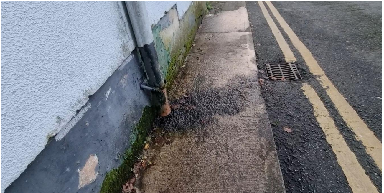
Figure 21: Existing Drains creating slippery conditions on St Patrickswell Lane Gully adjacent will be located in centre of new pedestrian circulation area
