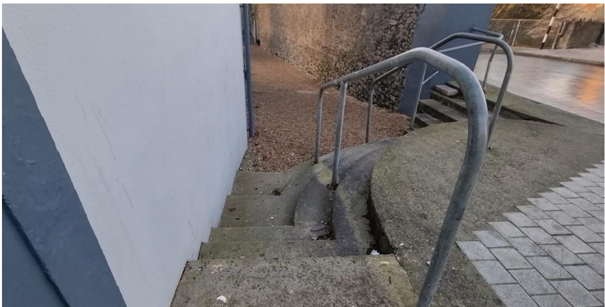
Figure 75: Narrow existing steps, No tactile at top and bottom
