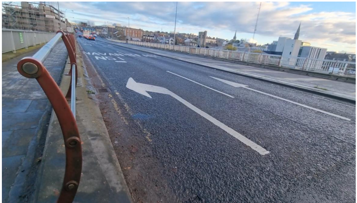
Figure 119: Old Road Markings to be Removed
