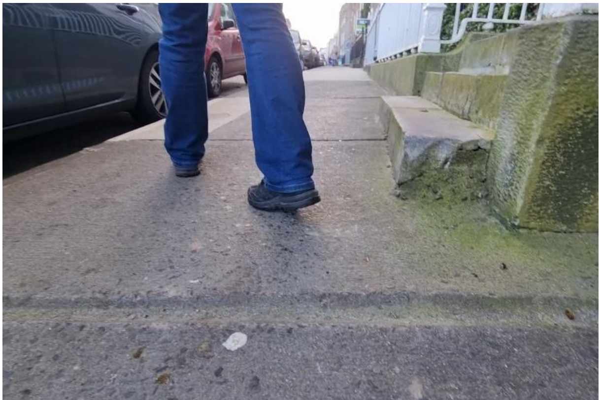
Figure 80: Steps presenting trip hazards in footways
