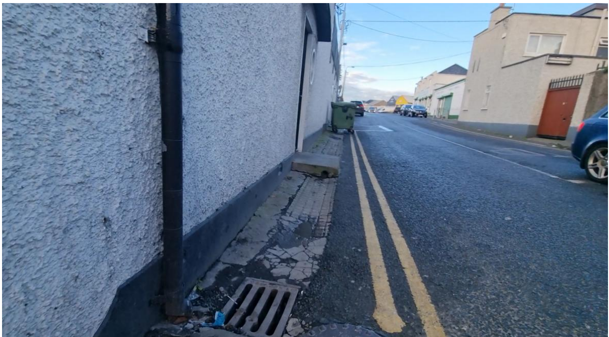
Figure 97: No footway at tie in on Fair Green
