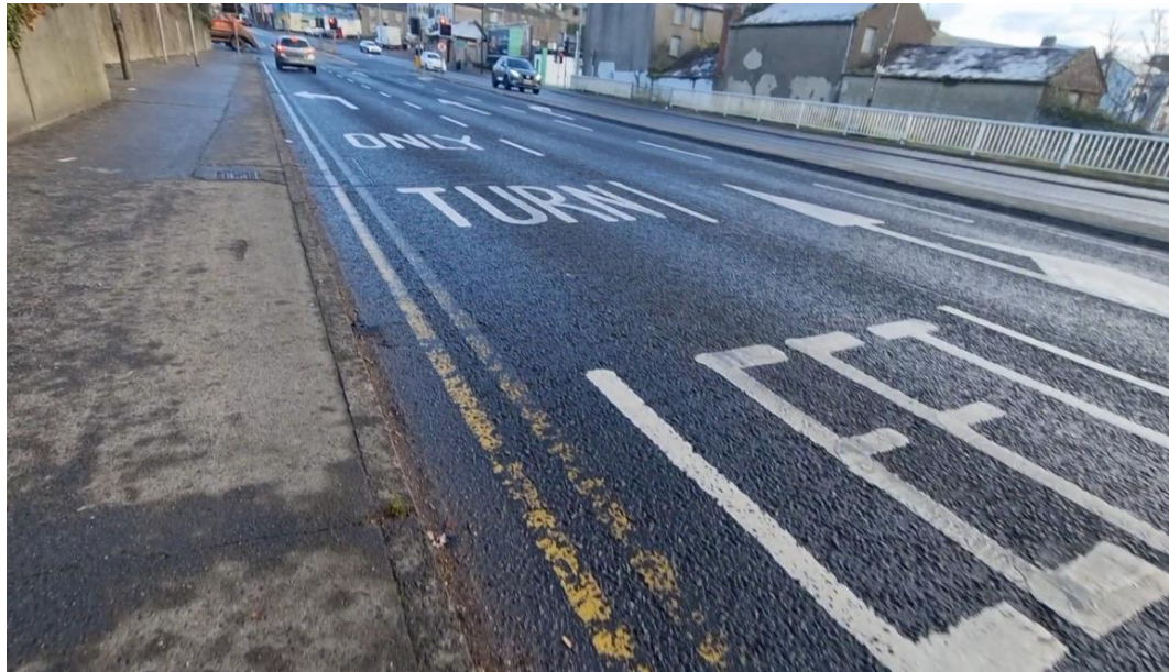
Figure 122: Redundant Road Markings
