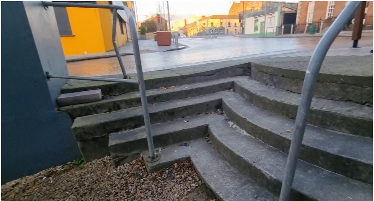
Figure 79: Existing non compliant steps and handrails
