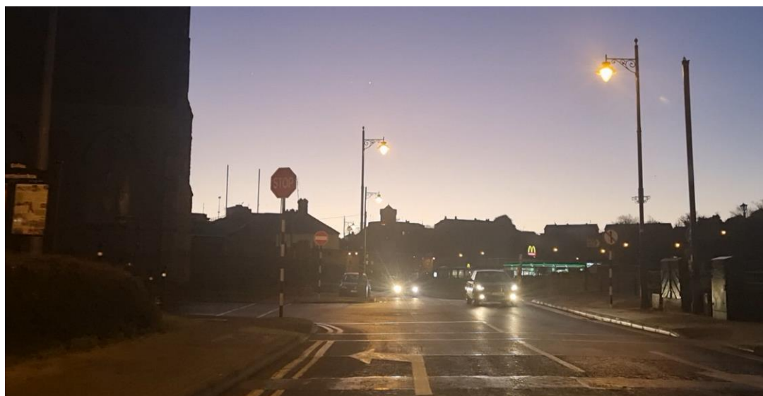
Figure 140: existing Stop Line & Sign removed at Intersection of Father Connolly way/Dominic Street?
