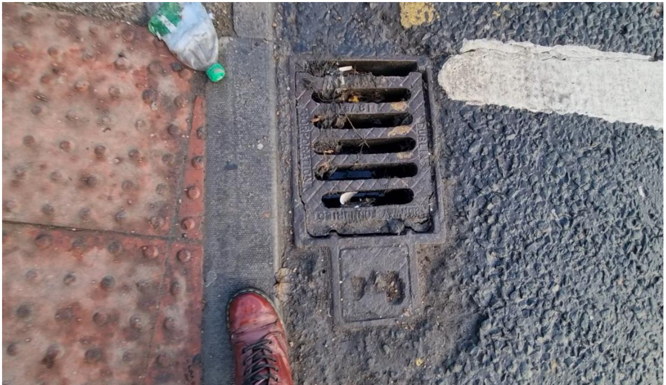
Figure 22: Gully in desire line at pedestrian crossing on George's Street
