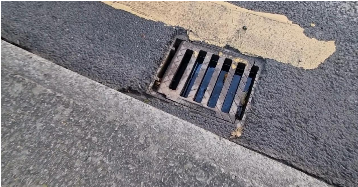
Figure 19: Existing Blocked Gully on Father Connolly Way
