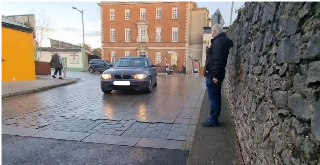
Figure 23: Pavement Damage at Transition between surface types
