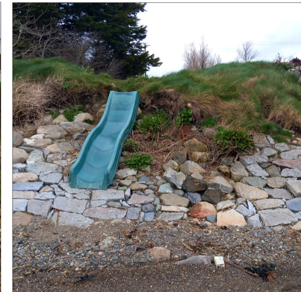
Image P2 - Existing coastal defence stonework displaced and non effective
