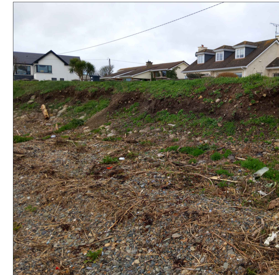
Image P1 - Eroding clay bank with no existing protection
