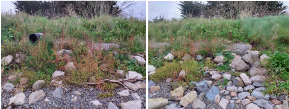
Plate 6. Two ground photographs taken on the 7 th October, 2023 at Chainage 205m to 220m facing in a north-westerly direction towards Location B proposed coastal works area showing concrete footing with collapsed stone sea wall beneath
