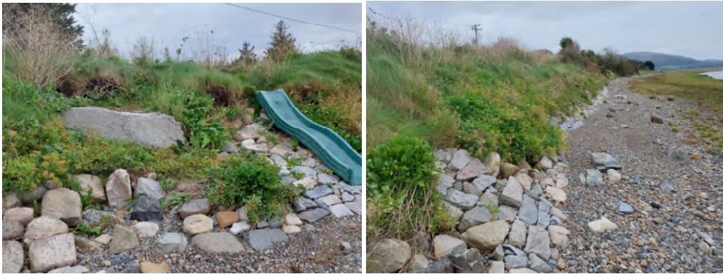
Plate 8. Two ground photographs taken on the 7 th October, 2023 at Chainage 220m facing in northerly and easterly directions towards Location C proposed coastal works area showing damaged stone sea wall
