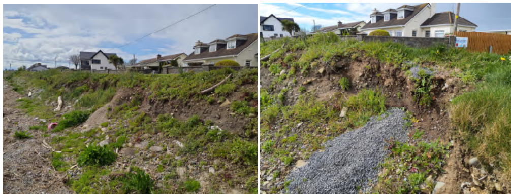
Plate 4. Two ground photographs taken on the 17 th April, 2023 at Chainage 30m facing in a north-westerly direction towards Location A proposed coastal works area showing damaged stone sea wall on the western side and soil collapse in the middle of Location A Works Area
