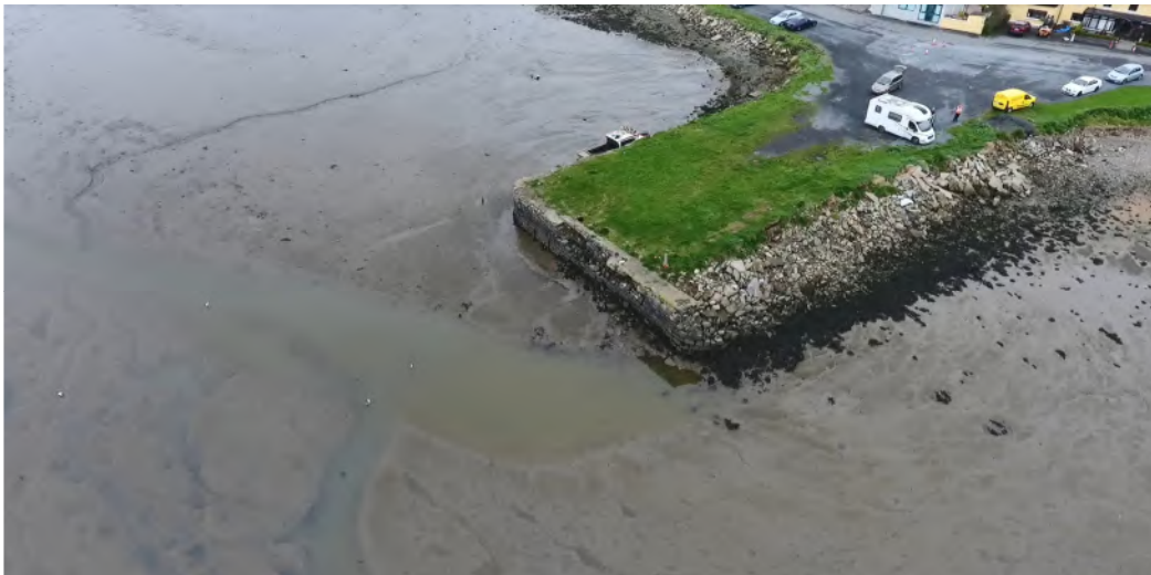
Plate 18. Aerial photograph taken at 30m elevation to the southeast of Bellurgan Quay facing in a north-westerly direction showing ponded stormwater from the stormwater outfall
