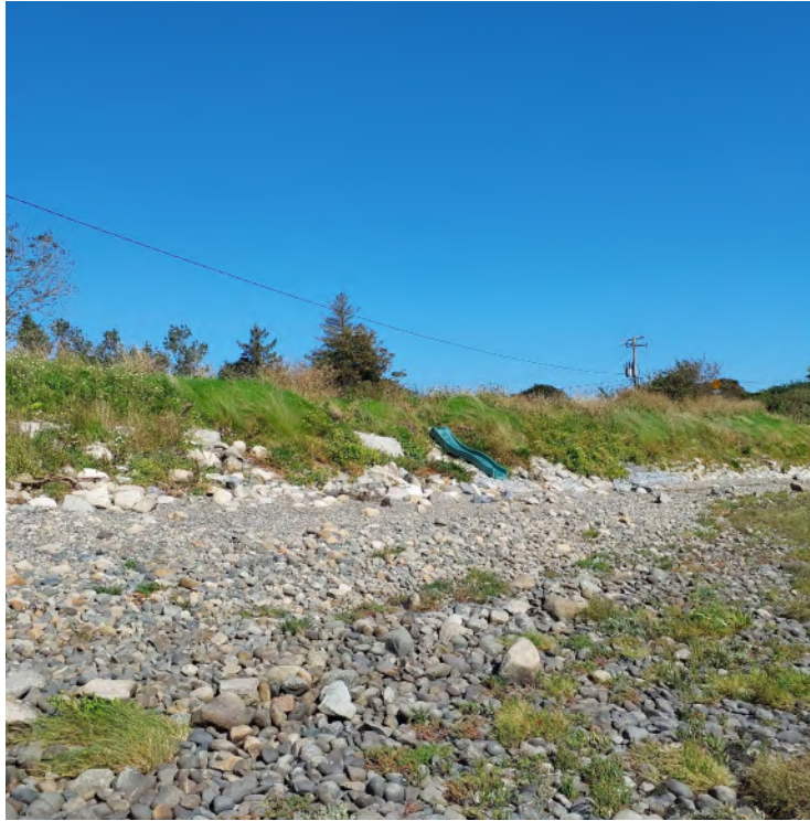
Plate 24. Ground photograph taken to the south of Location B works area facing in a north-easterly direction showing stone sea wall along Locations B and C work areas (i.e., Sea Walls, Piers, and Jetties (CCI) habitat )
