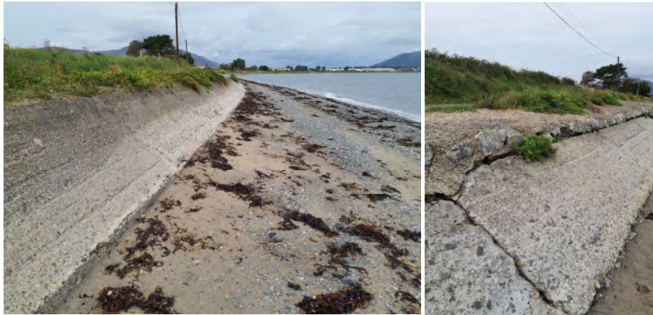
Plate 3. Ground photographs of seawall with crack caused by sea erosion
