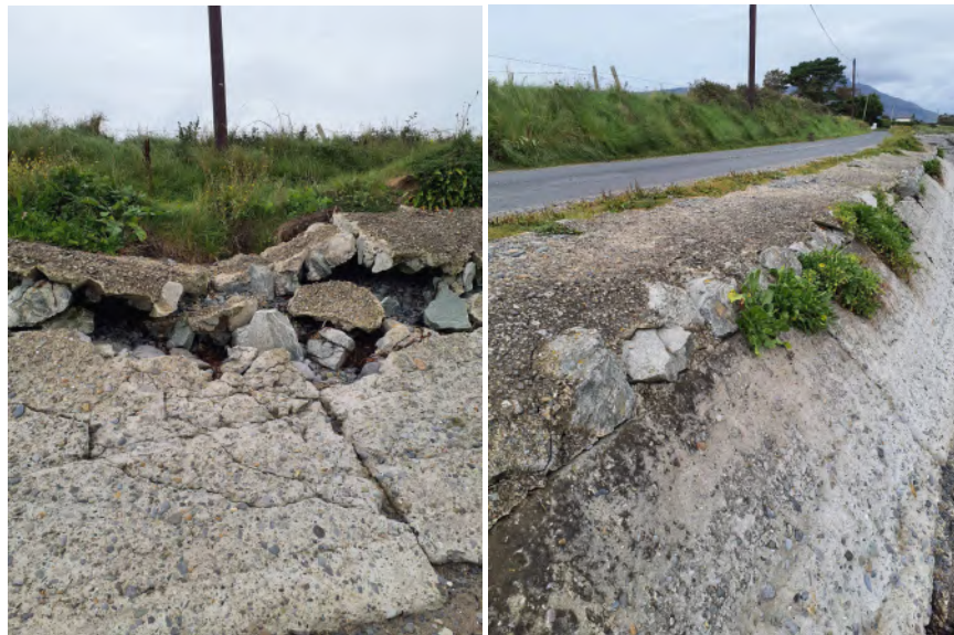
Plate 4. Concrete cap along seawall showing evidence of erosion at the cap seawall interface at the top and where the cap and seawall have collapsed exposing the gravel and boulder foundations to erosion
