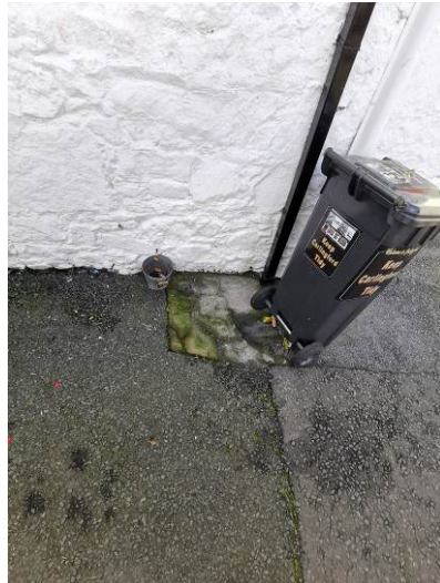
Plate 15 View of concrete covered area to north side of Bakers Street CH11, facing north
